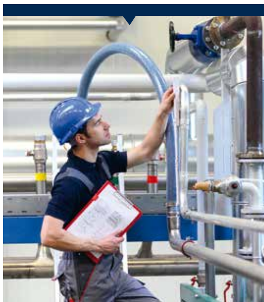
Process security is becoming ever more important in complex plants, where flexibility and cost-effectiveness are also crucial.
