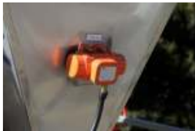
Vibrator on side of hopper
