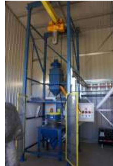
Crane and hoist bulk bag unloader or fork lift - bag unloader
