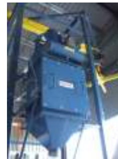
Dust extractor, valved between hopper and bag unloader
