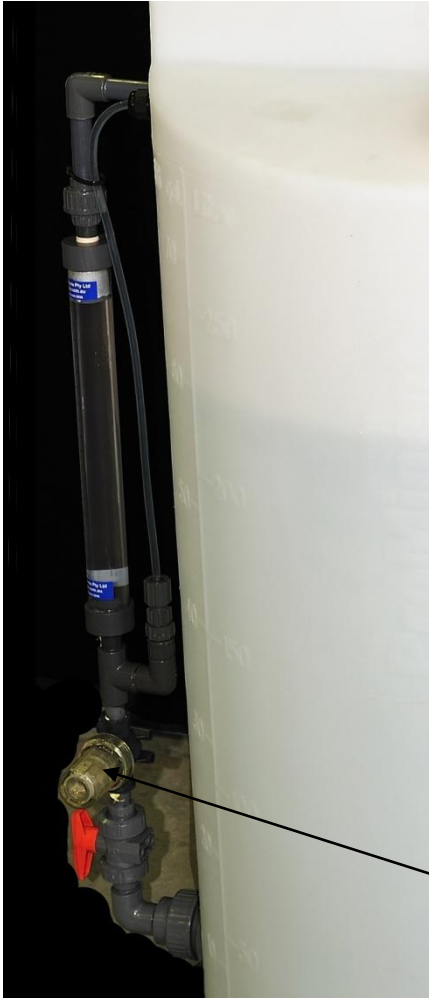
Suction pipework with filter, suction valve, calibration cylinder and isolation valve
